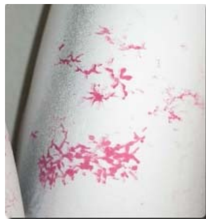
Indications of cracks on smelt spout tube
